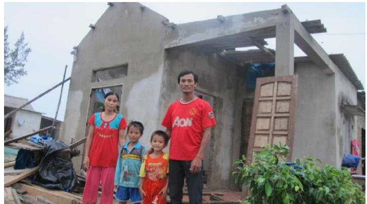
Unroofed and damaged house in Vinh Linh District in Quang Tri Province (JAT Quang Tri)
