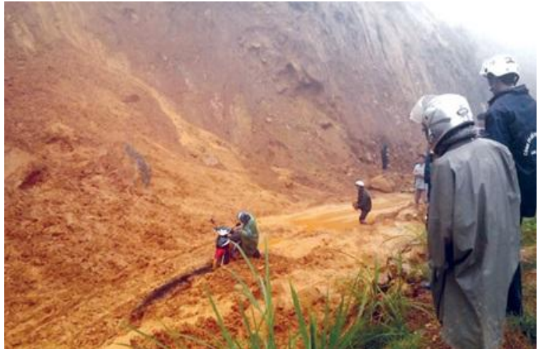
A landslide covers a road on the route from Lai Chau City to Sin Ho District. — VNA/VNS Photo Nguyen Cong Hai
